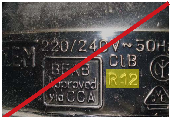
Refrigeration compressor with forbidden refrigerant
