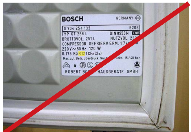
Refrigerator with forbidden refrigerant R12
